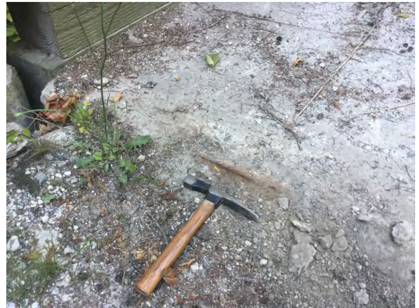
Damaged Girder End
