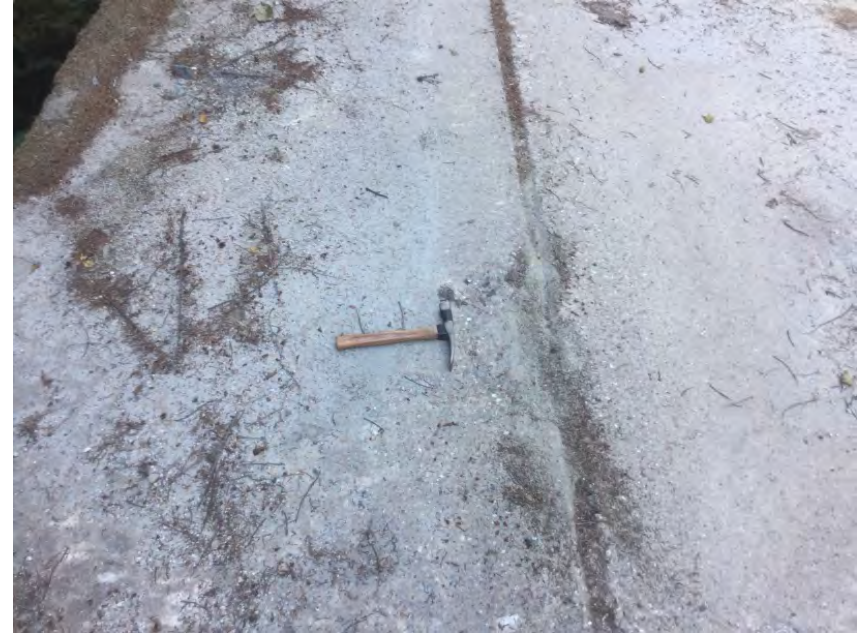
Spall in Deck
